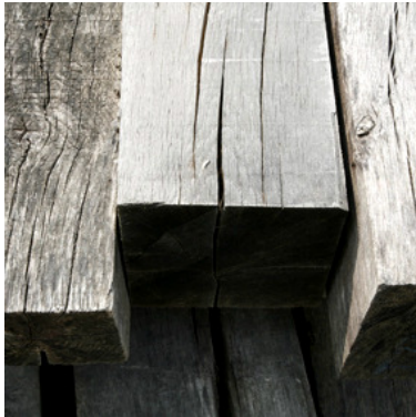
Seasoned beams, silvered down and opening up cracks & splits along the length
