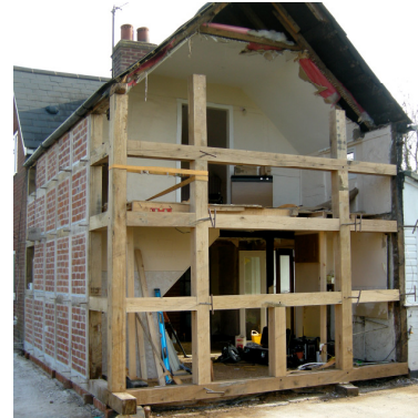
Beams air dried to a low ambient moisture content suitable for restoration projects
